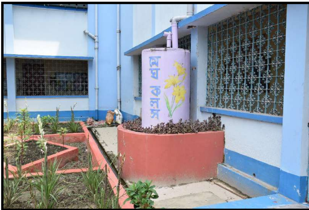
Plate 8: Rainwater Harvesting (Megh Kalas)
