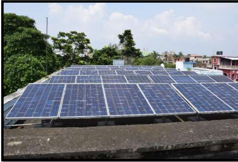
Plate 1: Solar power system for Green Energy
