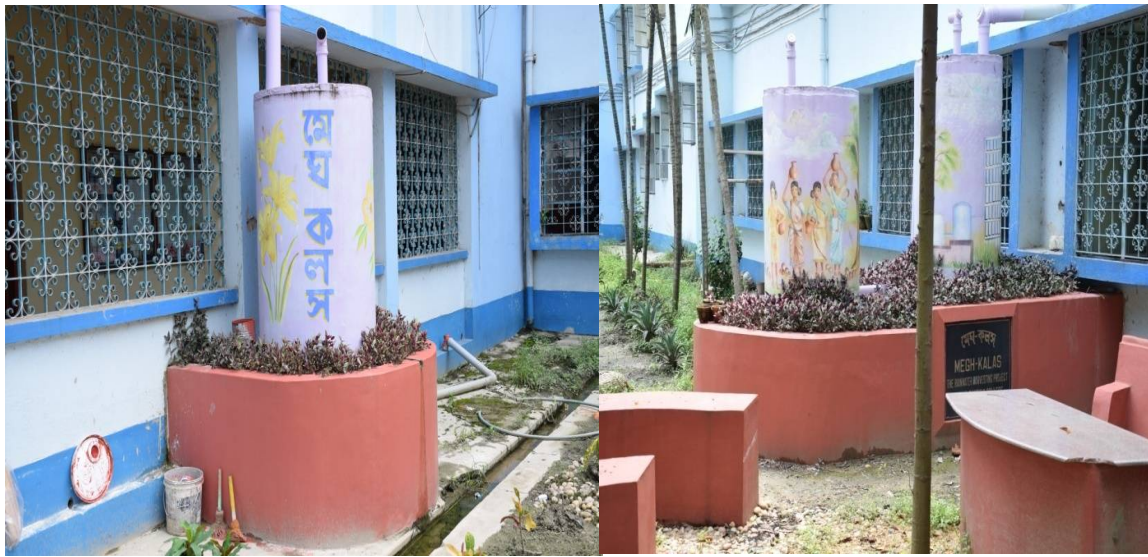
Figure 2: Rainwater Harvesting facility of the College
