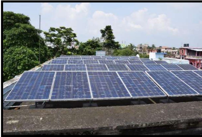
Plate 7: Solar power system for Green Energy
