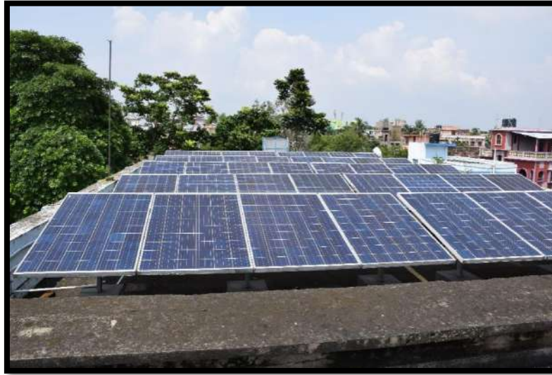
Plate 1: Solar power system for Green Energy
