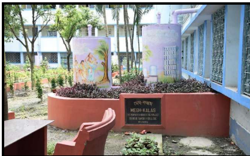
Plate 1: Rainwater Harvesting facility of the College
